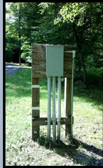
Loop II Breaker
